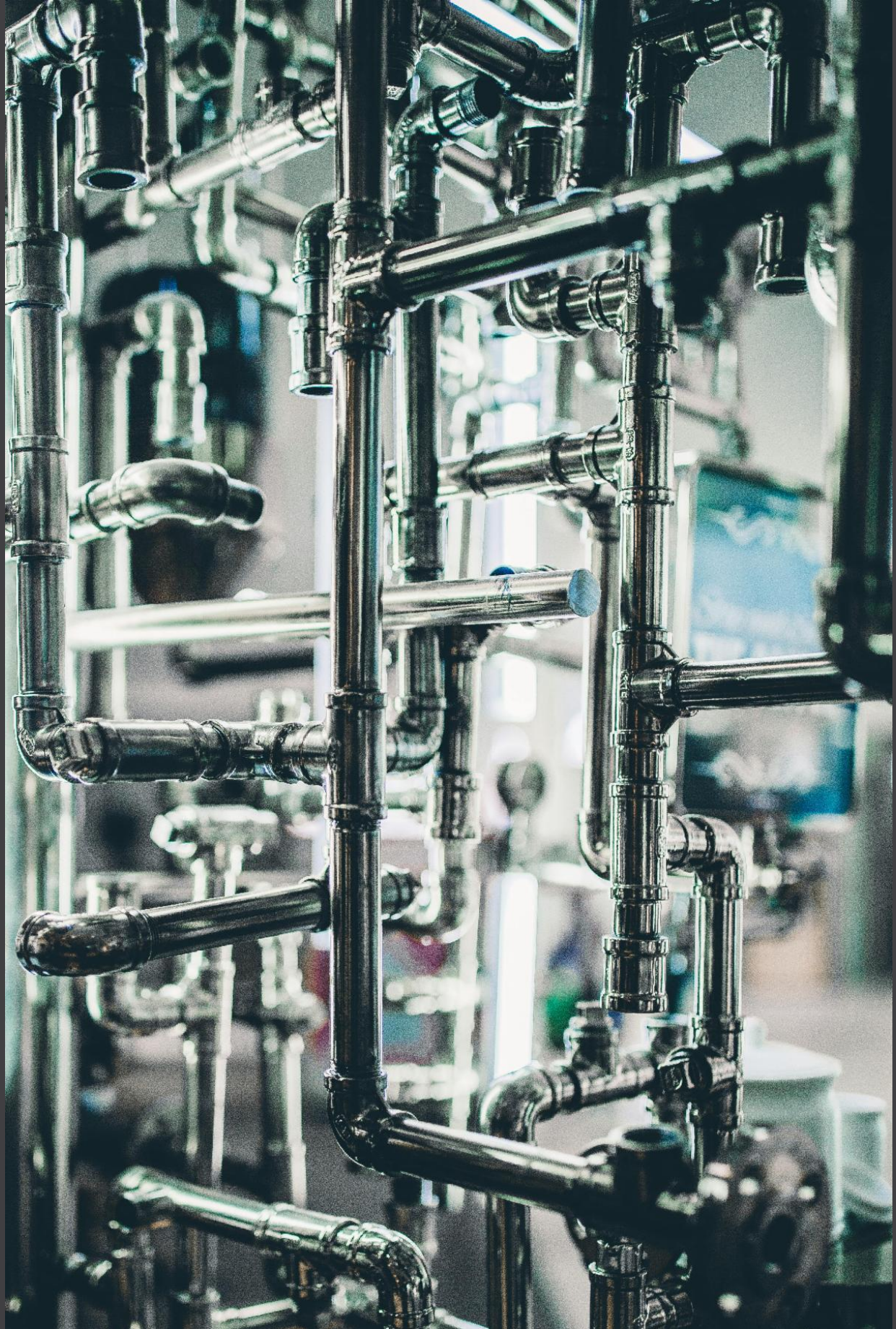
Chrome Pipe Lines By Jiawei Cui
